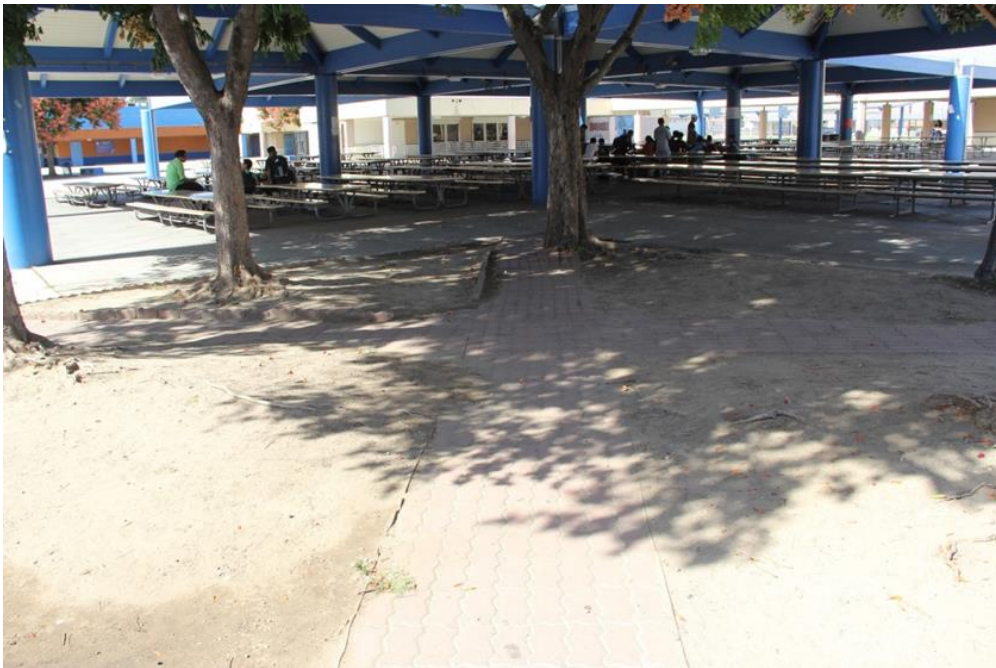
Trees Causing Uplift On Brick Pavers
